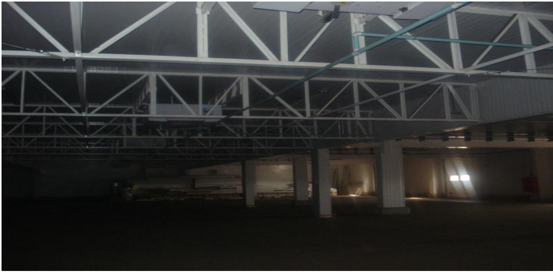
Figure 4. Cold storage room.
